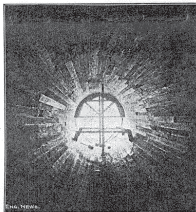
Fig. 3.—Interior View of 9-ft. Redwood Stave Pipe, Near Floriston, Cal.
