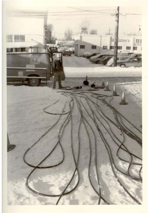
Figure 11. Early Inspection Cable arrangement Source: Pipe Recon Services, Surrey, BC.
