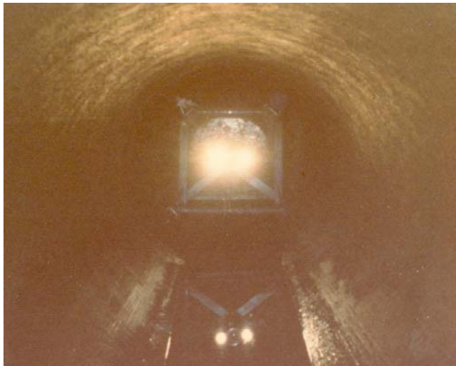
Figure 7. Early inspection camera, in 36" Trunk line Source: Pipe Recon Services, Surrey, BC.
